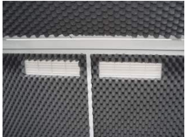
Sound proofing inside walls
